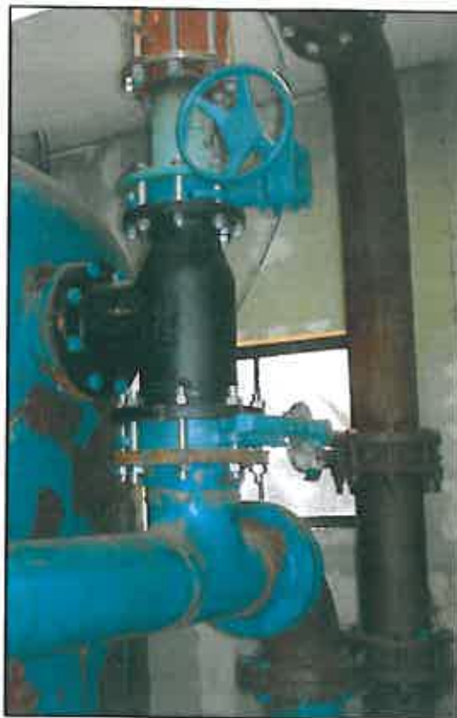
Figure 7: NEW Filter Valves
